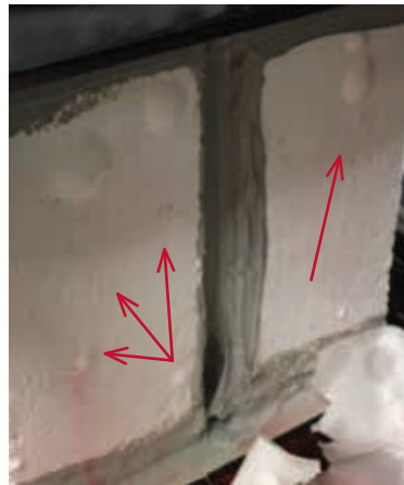
Bottom right: Performance of commercial quality exterior residential paint under hydrostatic pressure. Blisters formed at 4psi, failing ASTM D 7088 test.
