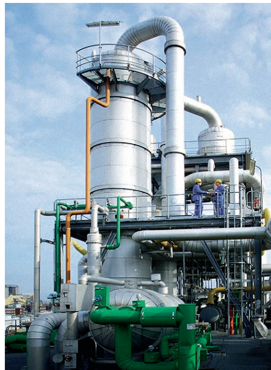
Almost 30 years of top-level PolyTHF production: the PolyTHF facility at BASF's integrated "Verbund" site Ludwigshafen, Germany. Besides, BASF is producing PolyTHF at three other plants in USA, China and Korea.
